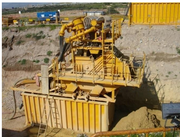
Separation plant for extracted material.
