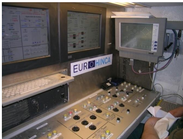
Control cabin of an EPB TBM
