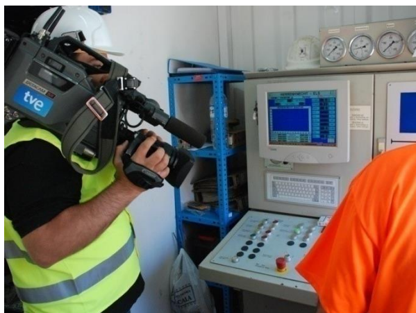
TBM control panel located on the surface.
